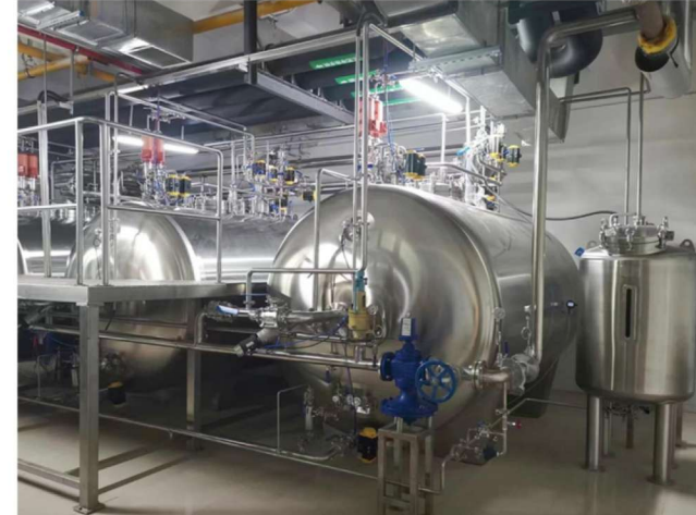
废水灭活系统 Wastewater Inactivation System
